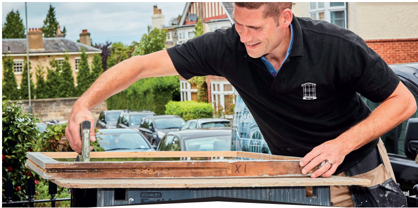
The new, high performance 12mm double glazed unit is installed into the sash.
