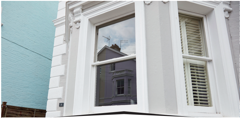
A typical single glazed, draughty, Victoria Sash window, which needs restoration.
