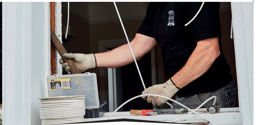
The sash is weighed and the frame re-corded and re-weighted to ensure the correct operation when fitted.
